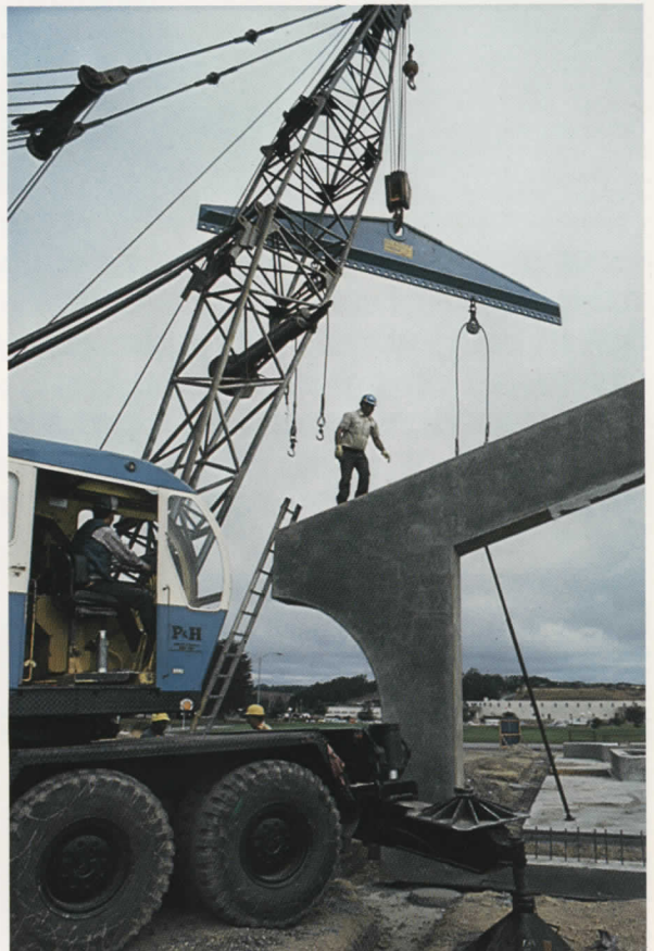
The walls went up on Intel's Santa Cruz facility in August. The facility is now in full production.
